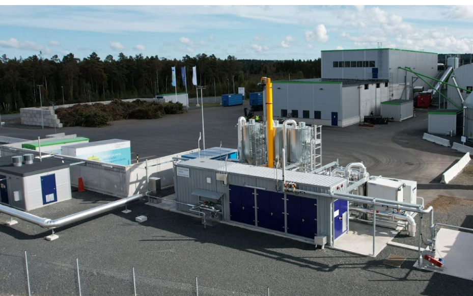
Jönköping/SWE: Komogas® plant with membrane gas upgrading for fuel production (CBG/BioCNG)
