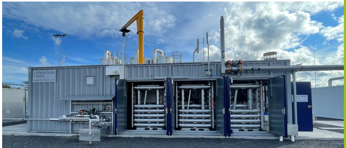
Gas upgrading plant with membrane technology
